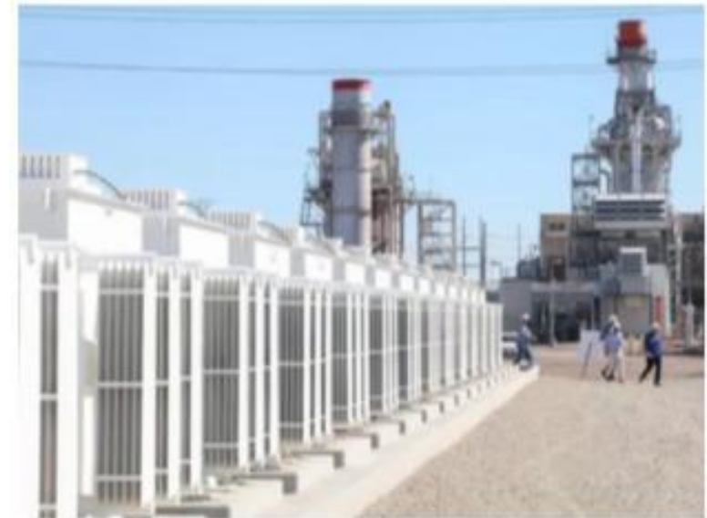
Imperial Irrigation District (IID) 30MW, 20MWh BESS project
