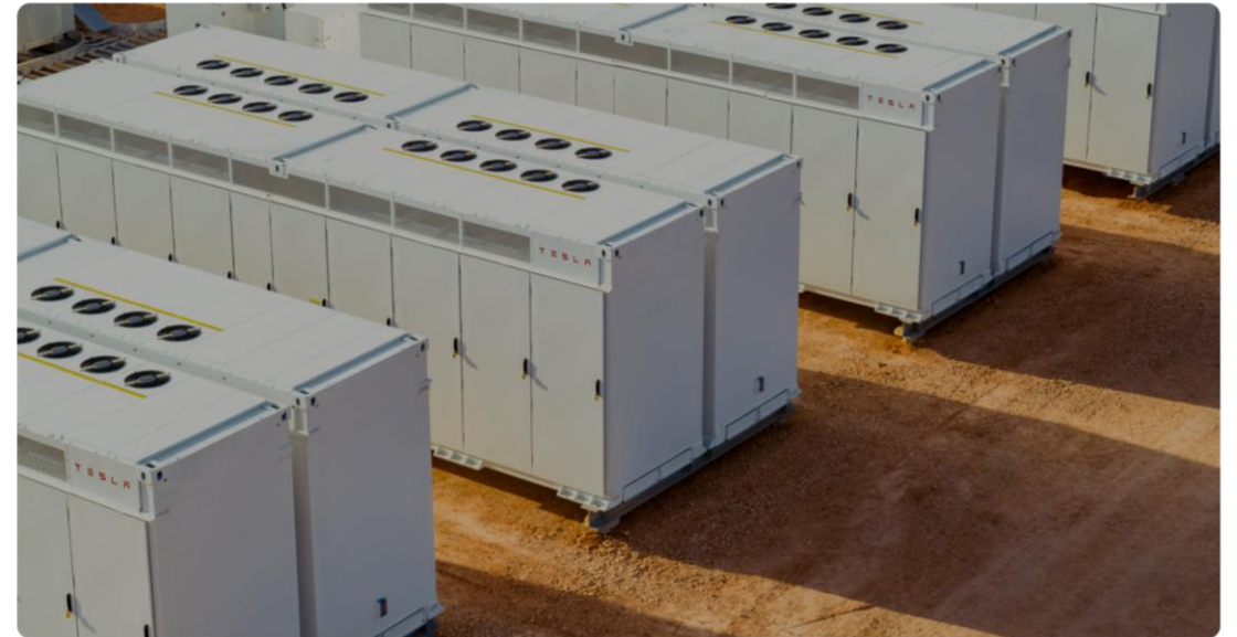
*Megapacks pictured not from project discussed on this slide
