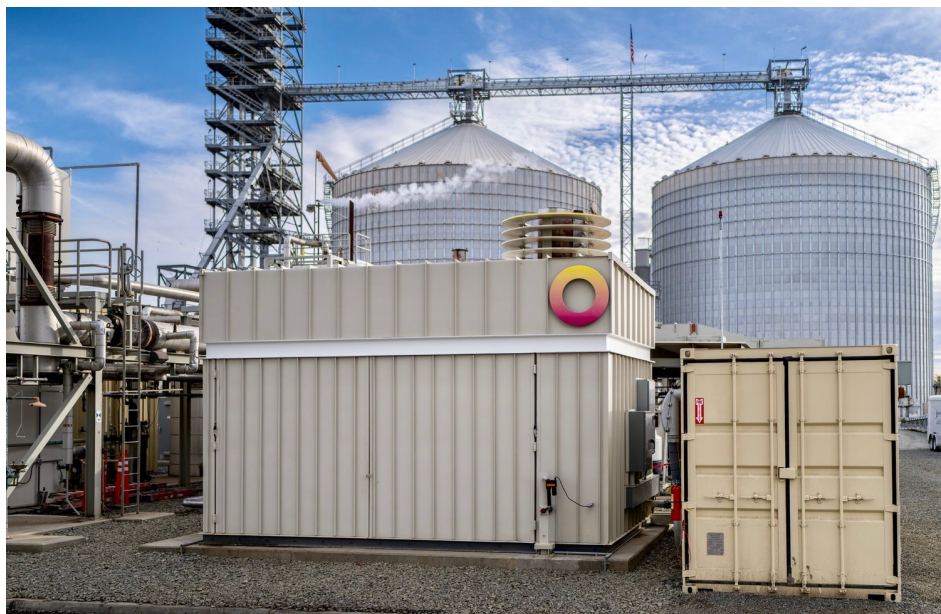
Pilot - 2 MWh Operating
