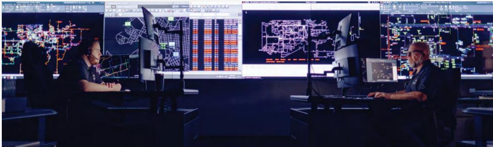
GrandBridge Energy System Control Center
