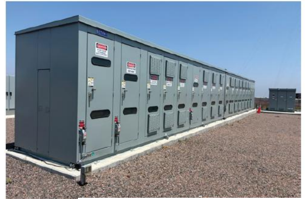
Source: Shahil Shah, National Renewable Energy Laboratory.
