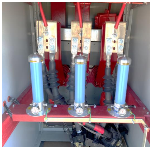
Resistive voltage divider and LEM sensor installation – Robb Wallen / NLR
