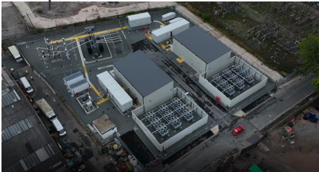
Lister Drive greener Grid park (Liverpool, UK). ABB's synchronous condensers with flywheels. Photo courtesy: Statkraft
