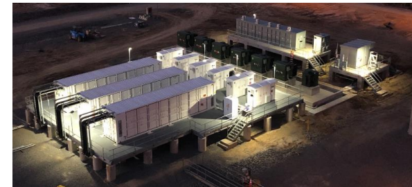
Entergy Perryville (complete, COD 4Q2019)
