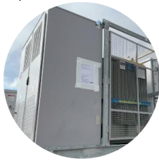
Inverter system (SMA)
