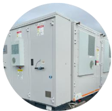
Battery system (Wartsilla)
