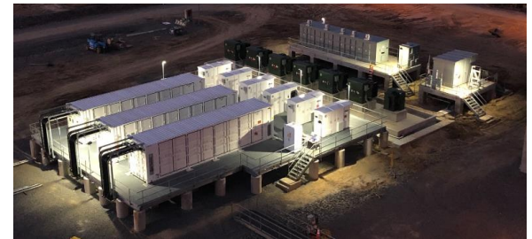
Entergy Perryville (complete, COD 4Q2019)
