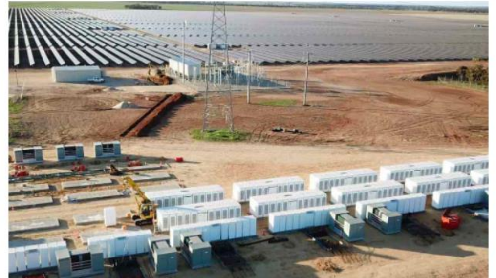
Gannawarra solar farm and battery storage facility. Source: Wiresol
