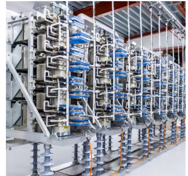
South Fork Offshore Wind GFM STATCOM
