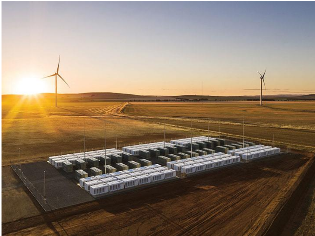
Figure 6: The world's largest Li-ion battery installed in South Australia, 100MW/129MWhr
